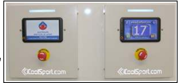
A Twin Remote Touch Screen Installation
